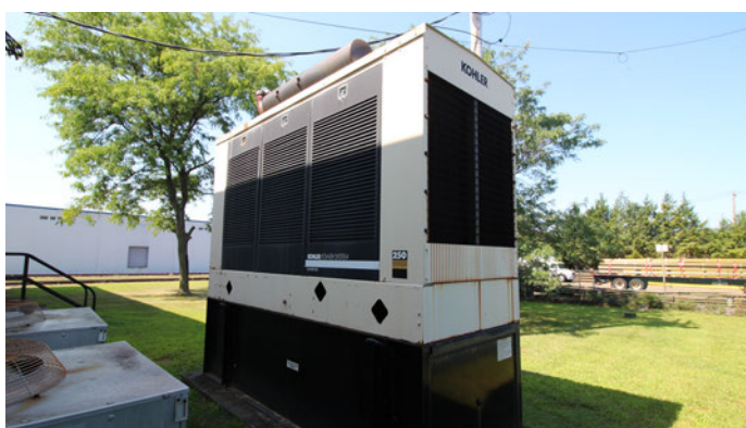
DECOMMISSIONED KOHLER 250 GENERATOR
