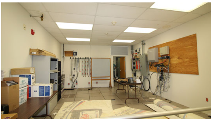
IT ROOM WITH RAISED FLOOR
